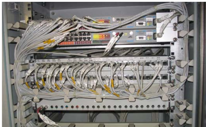
Fig. 2 Ethernet switch in the typical Control Network on a ship
