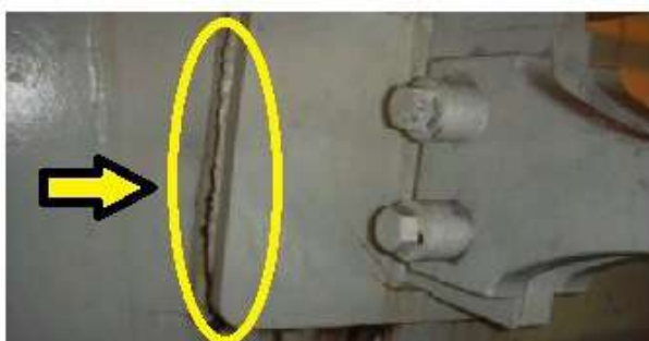
Top bracing detached from hull
