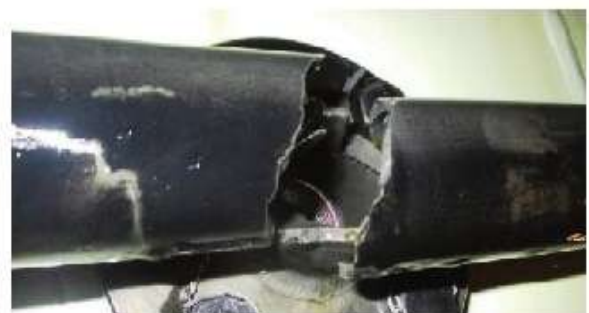
Ruptured lube oil pipe in Chain Casing
