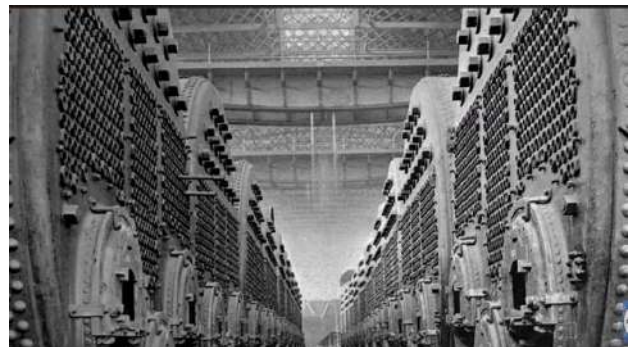
15 ft diameter, 20 ft long boilers - 29 of them
