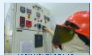
HIGH VOLTAGE LAB
