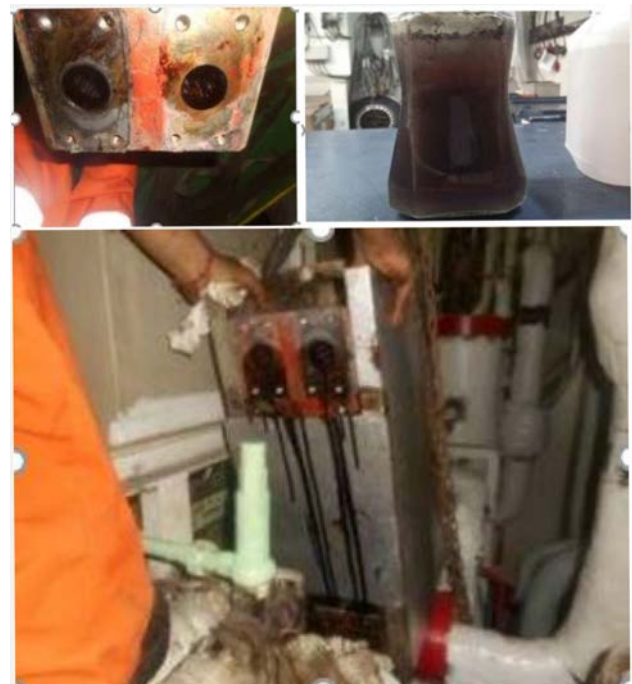
Figure 2. Fuel leak in heat exchanger & boiler water sample showing extent of oil contamination in the system
