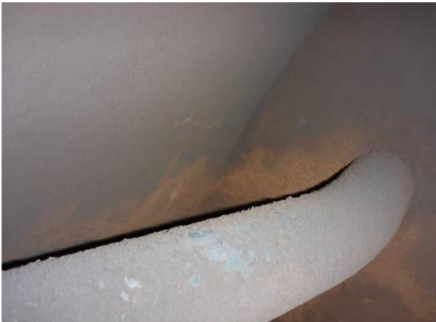
Figure 3. Thin barely visible Oil film adhering to outside of smoke tubes
