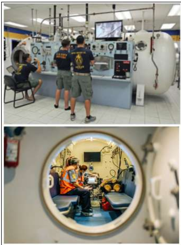
Figure 5. Deck Decompression Chamber
